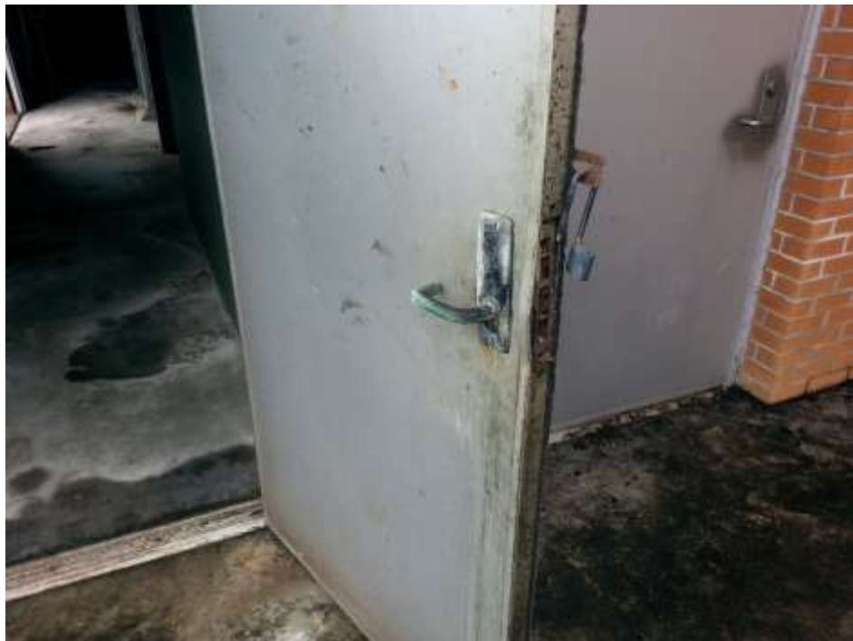
Photos 1 and 2 – Door threshold and corroded latch/lock set at the Screen Room
