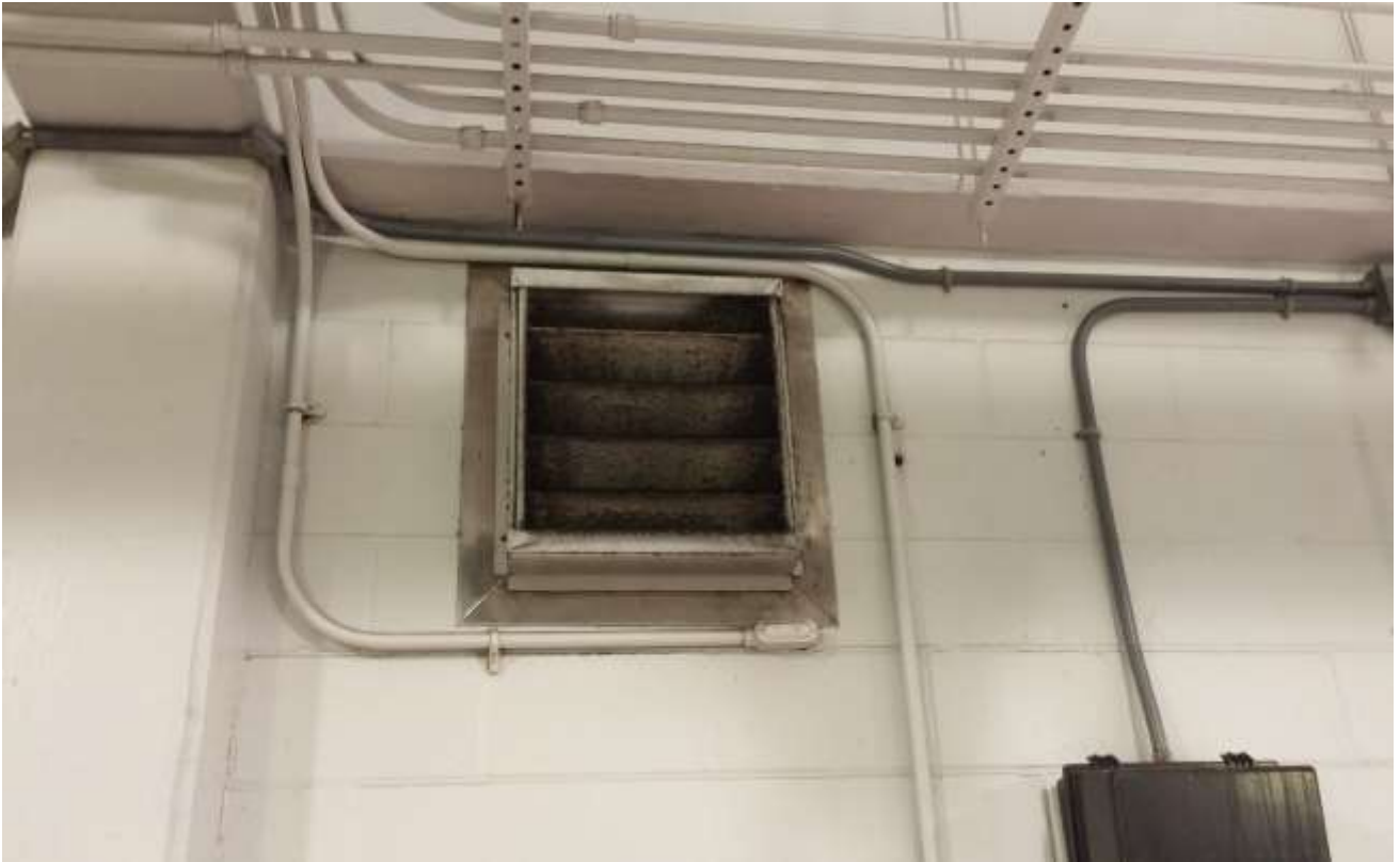
Photo 3 – Ventilation Fan to be replaced in-kind
