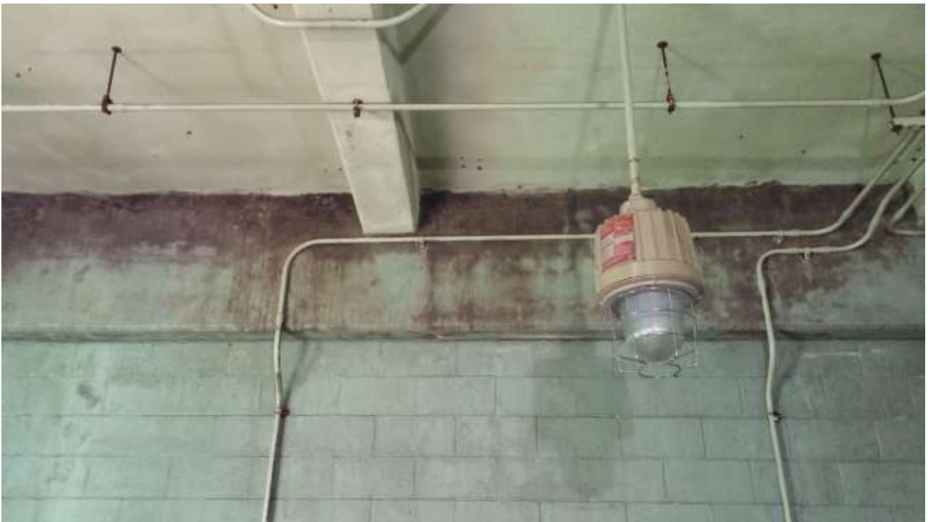
Photo 4 – Non-working Light Fixture
