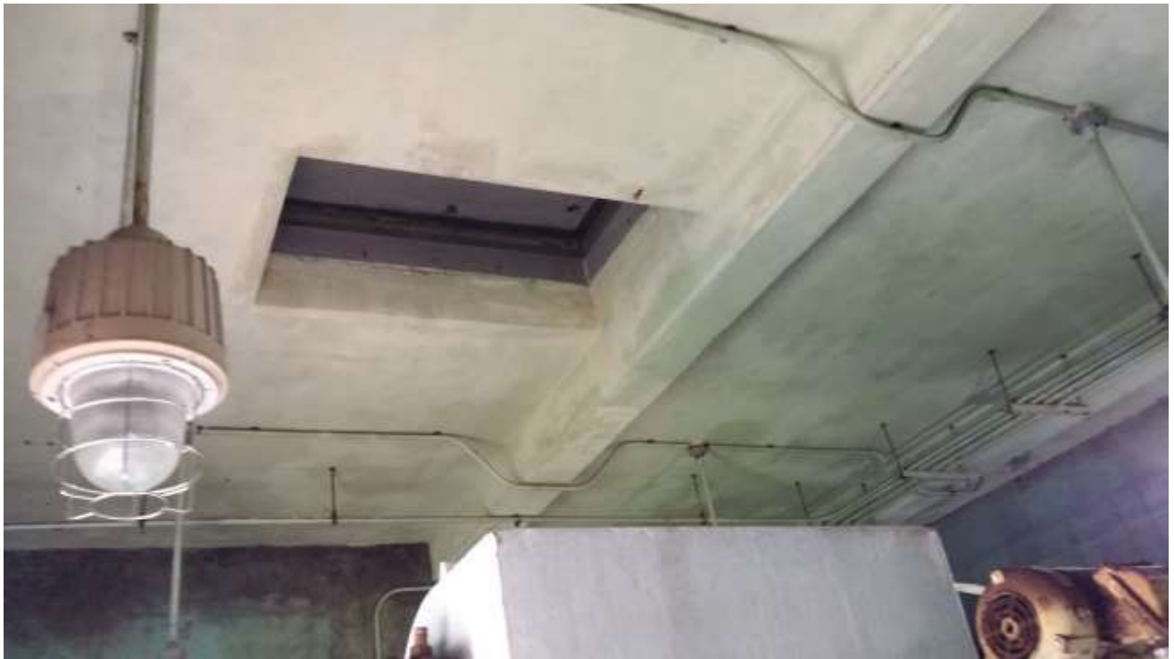
Photo 5 – Non-working Light Fixture
