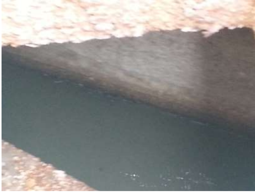
Photo 11 – Degraded concrete in the influent channel as seen from exterior concrete box.
