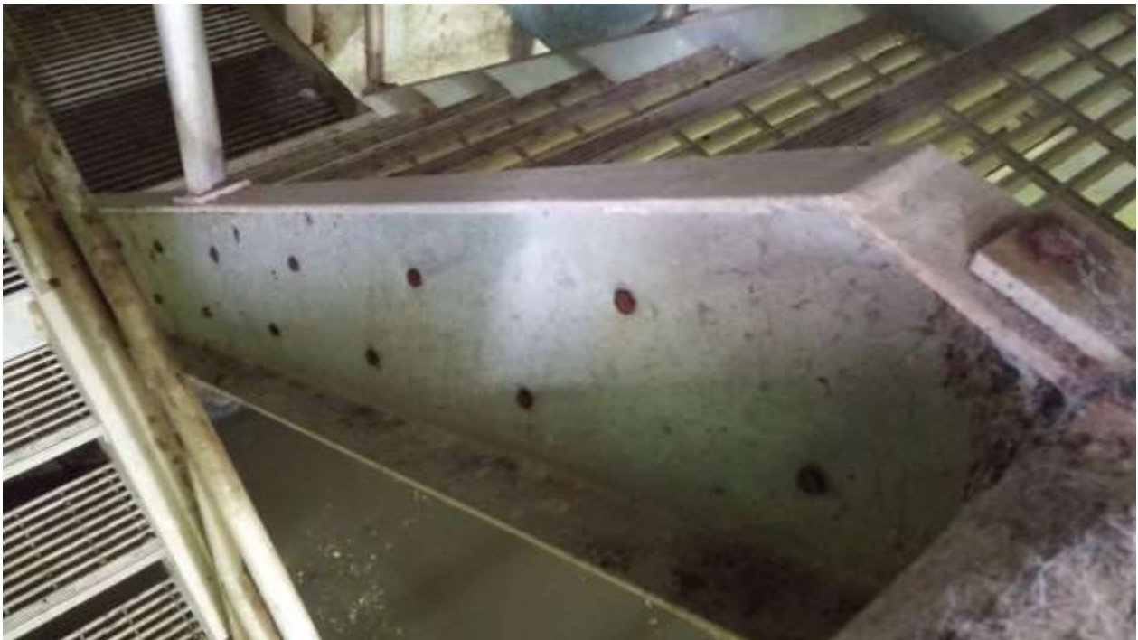
Photo 8 – Corroded Stairwell Bolts
