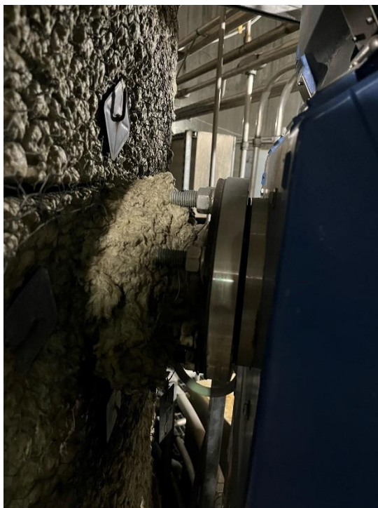
Figure 6: N02 Stack Sample Port Flange which is the same as N01
