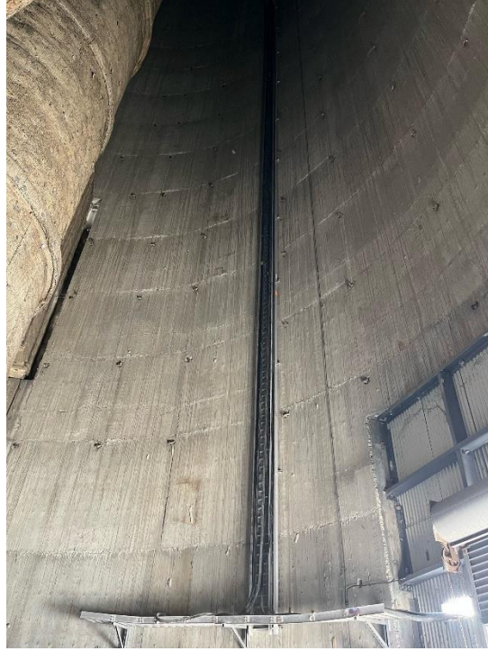
Figure 3: N01 and N02 Stack Umbilical Tray Inside of Stack
