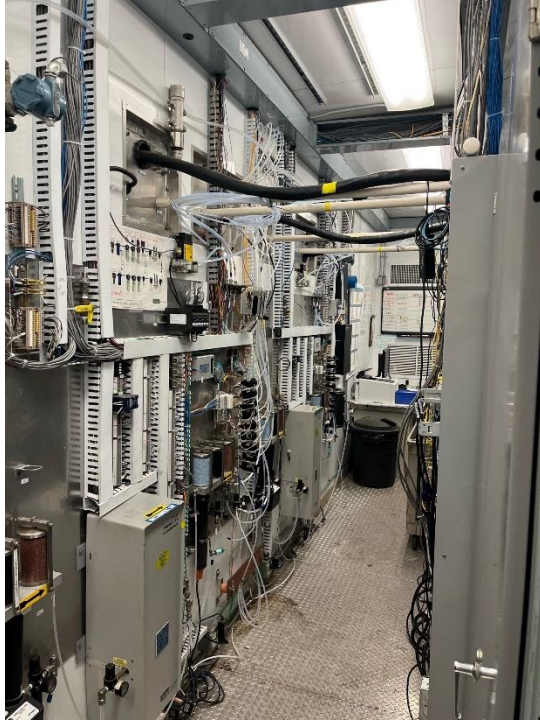
Figure 9: N01 and N02 Backside of Analyzer Racks and Umbilical Entries into CEMS Shack
