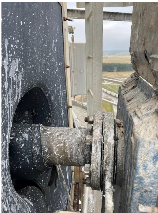
Figure 8: N03 Stack Sample Port Flange
