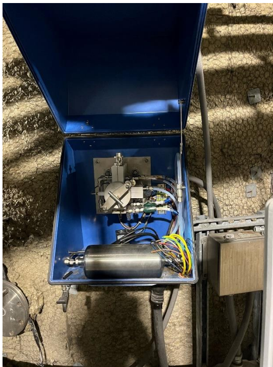
Figure 5: N02 Stack Sample Port which is the same as N01
