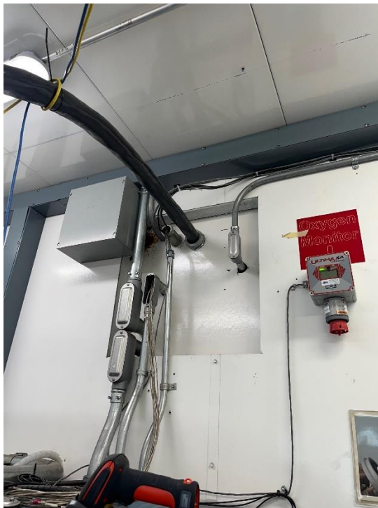
Figure 10: N03 Umbilical Entry into CEMS Shack
