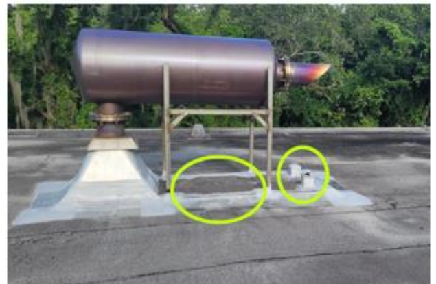
Existing concrete curb below generator exhaust to be covered with new roof and legs liquid flashed. Holes at leg tops to be fill with foam and capped. Thimble portion to be liquid flashed.
