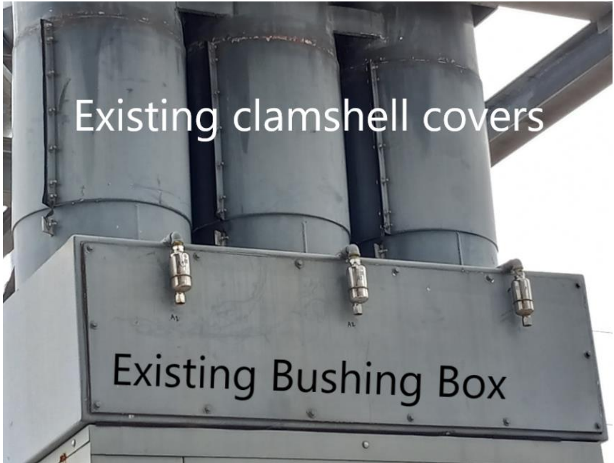
Existing clamshell covers on top of existing bushing box.
