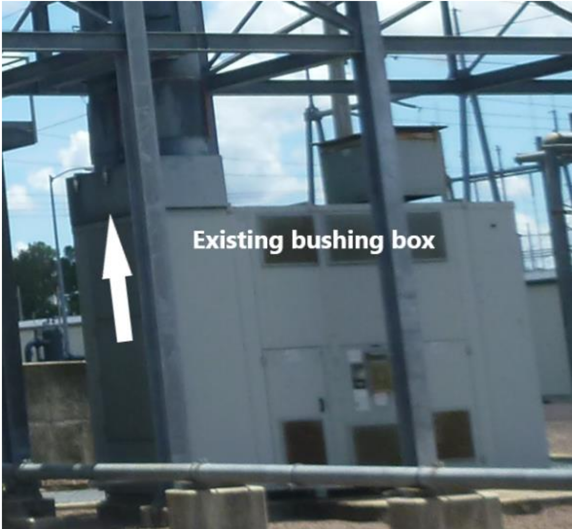
Profile of transformer pointing out existing bushing box.
