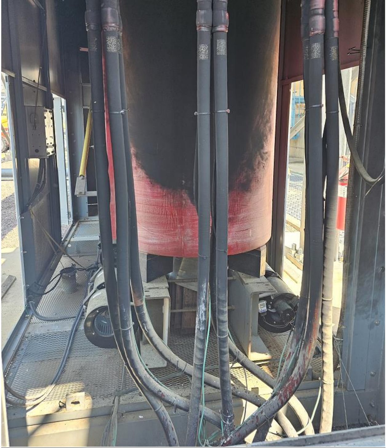
Secondary Medium Voltage 750MCM Cables.
