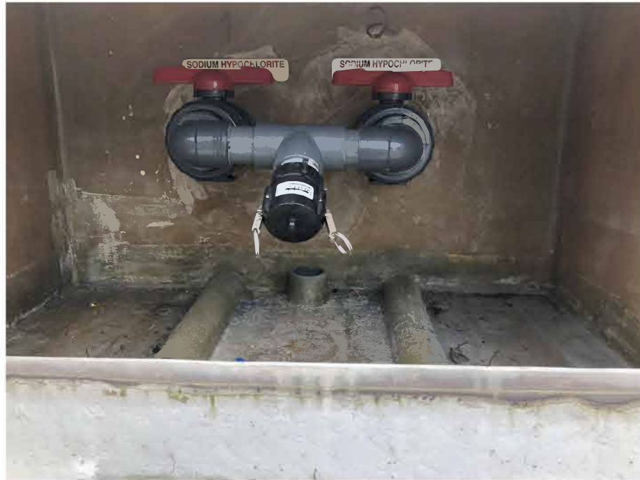
CHEMICAL FILL STATION PIPING
