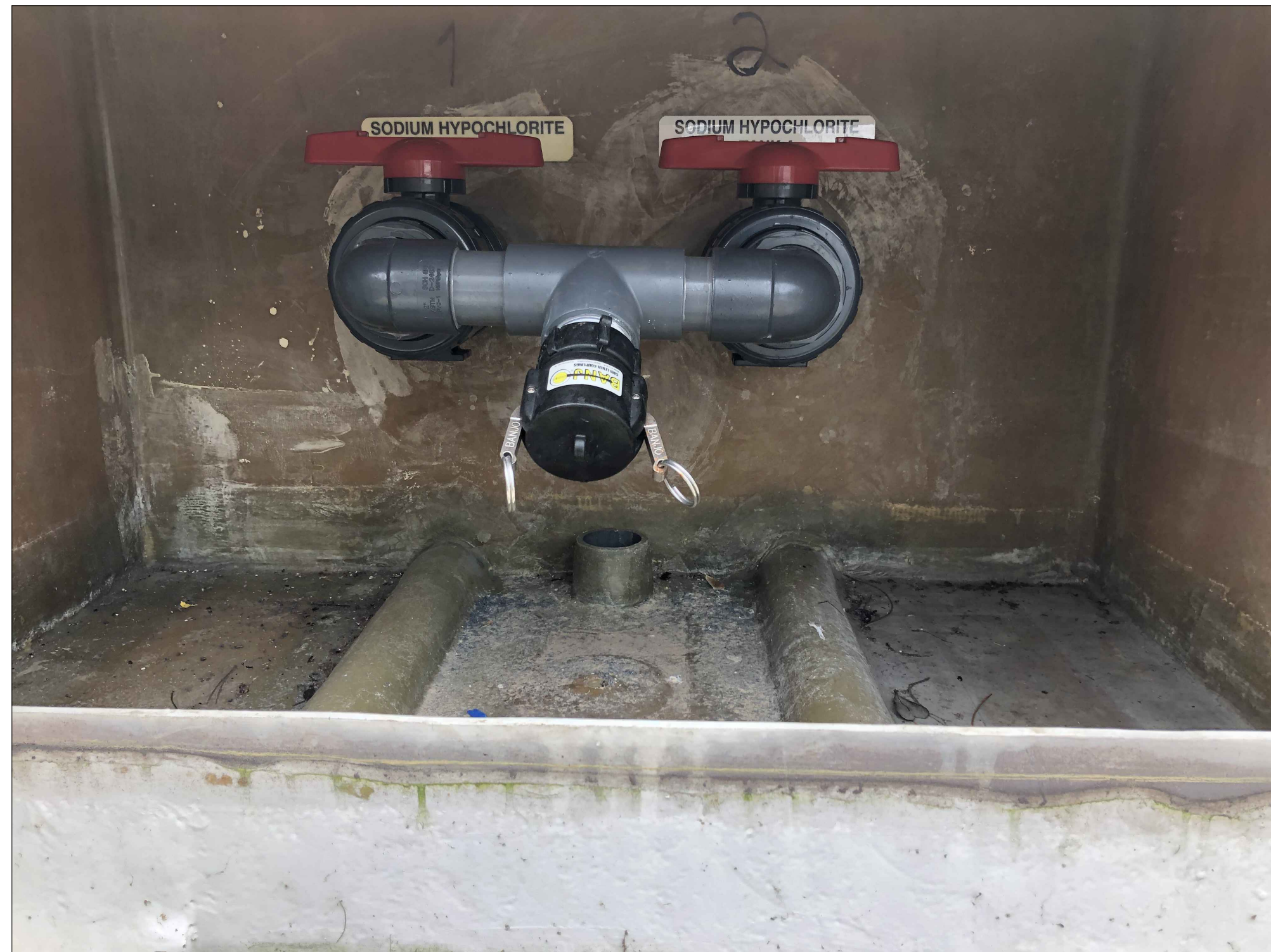
CHEMICAL FILL STATION PIPING
