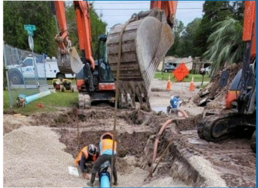
Hurricane Ian: 8" water main on the west side
