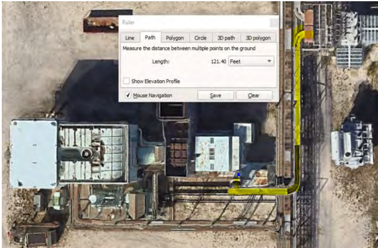
Cable Tray visible on Google Earth.
