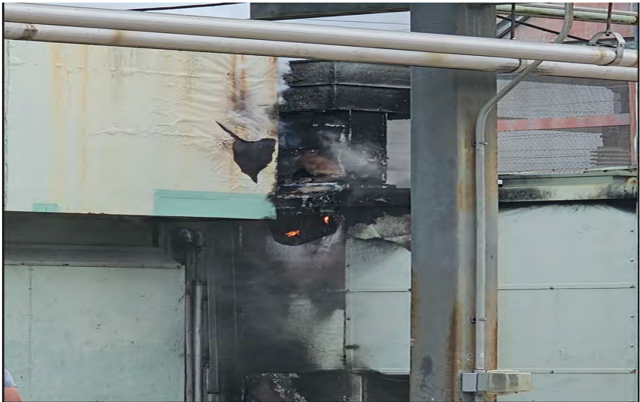
CT3 Catastrophic Damage.
