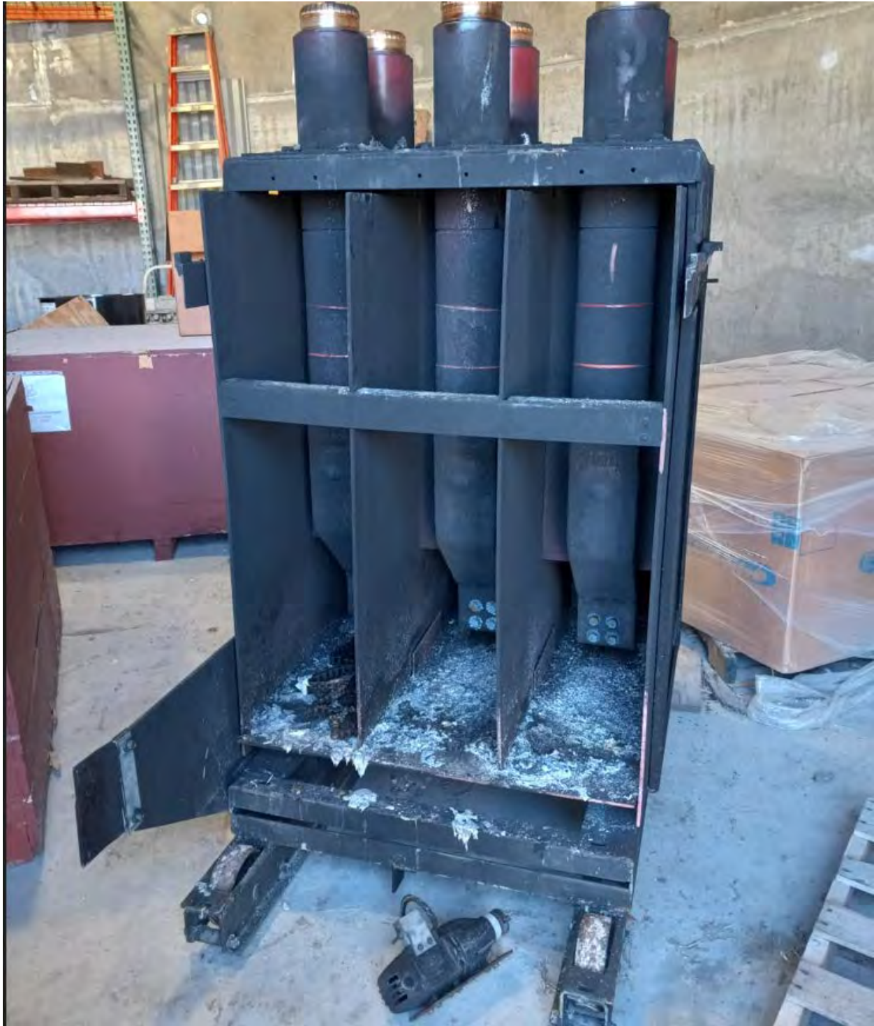
CT3 Catastrophic Damage.
