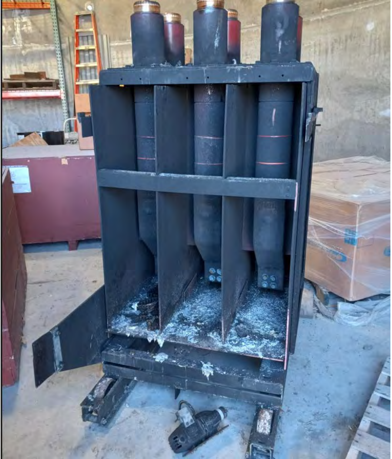
CT3 Catastrophic Damage.
