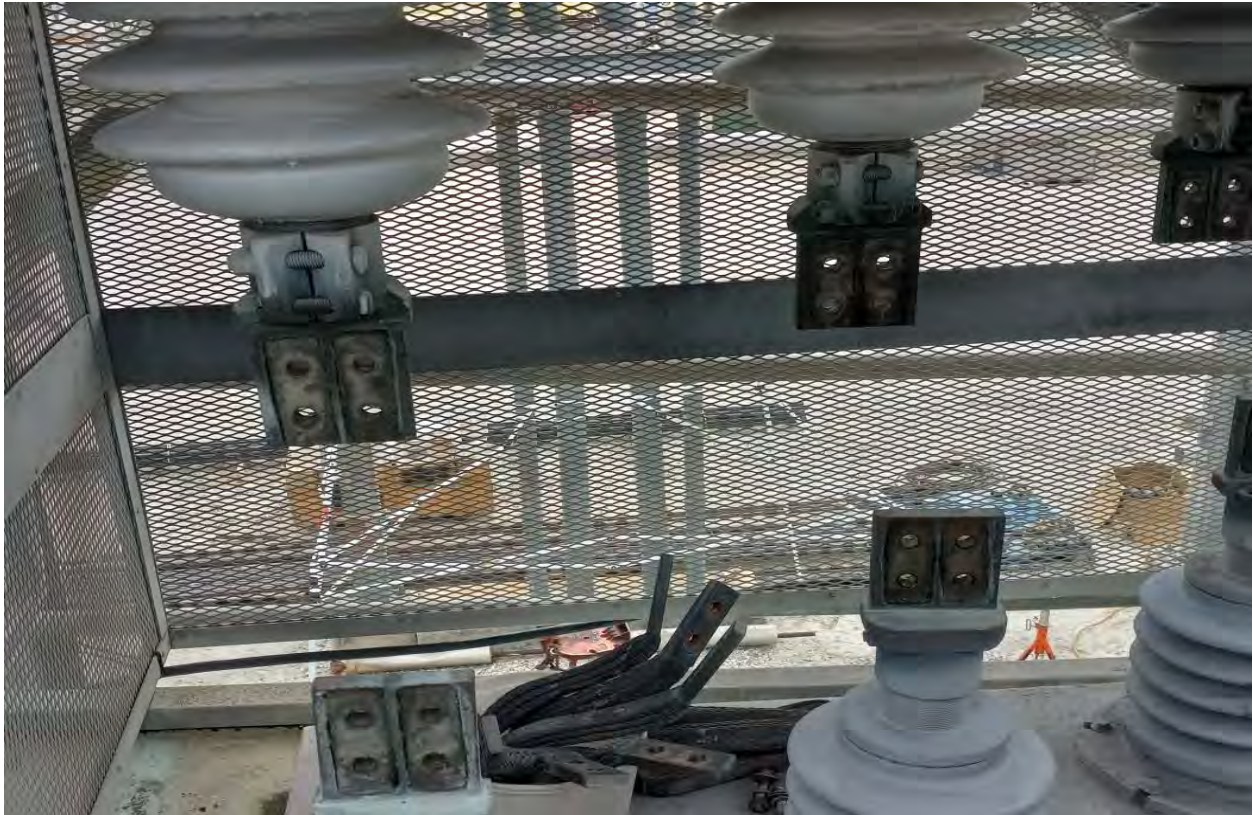
Top and Bottom Bushings at Generator and View of Eleven Inch Flex Links.
