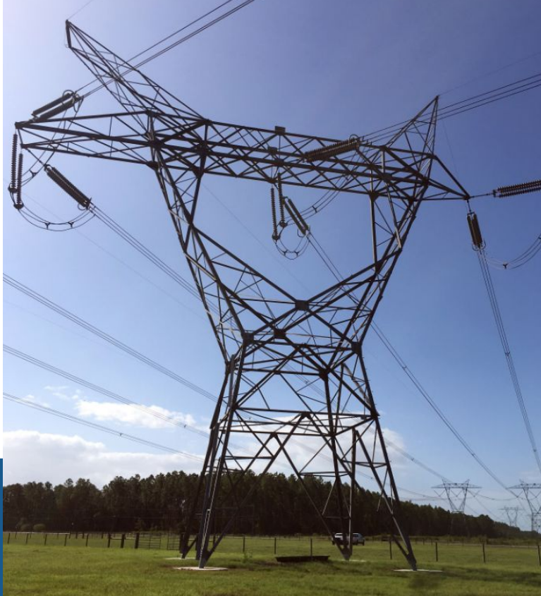
JEA Highspeed Transmission Line
