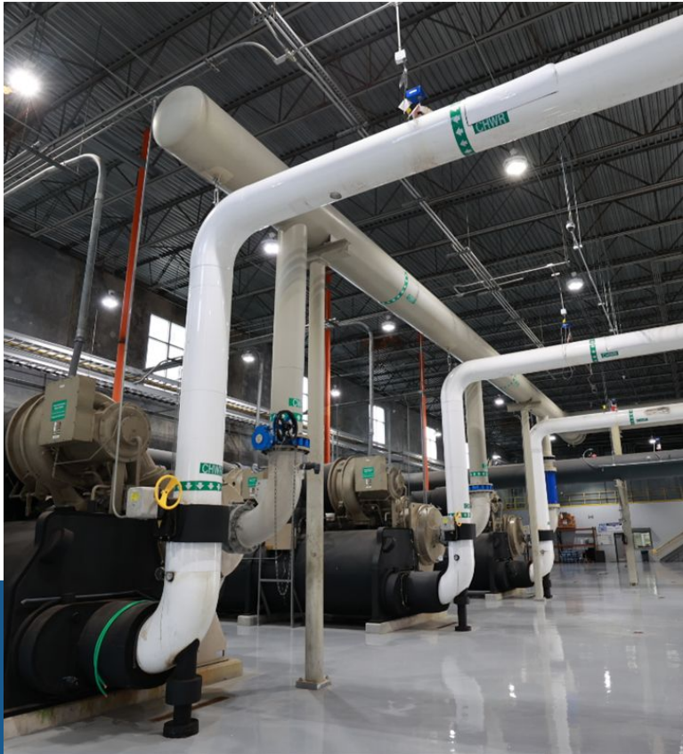
District Energy Systems Chilled Water
