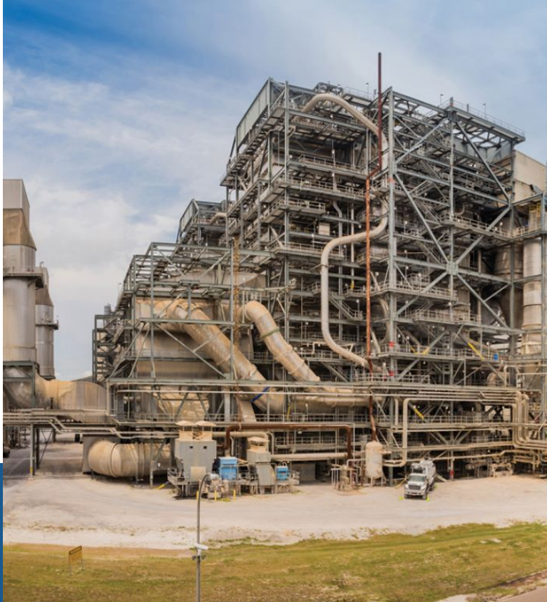
JEA Northside Generating Station
